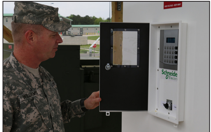
Brig. Gen. Timothy P. Williams, the Adjutant General of Virginia, prepares to symbolically turn the switch to send power from the solar array to the administrative and classroom facilities at the 183rd Regiment, Regional Training Institute.
