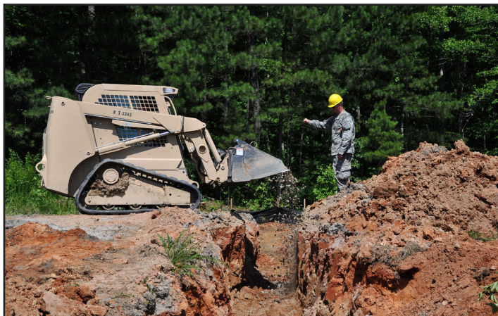
Virginia Guard engineers prepare to install culverts June 25, 2013, at Fort Pickett, Va. The engineers worked to improve roads and install new culverts along Fort Pickett's roadways.
